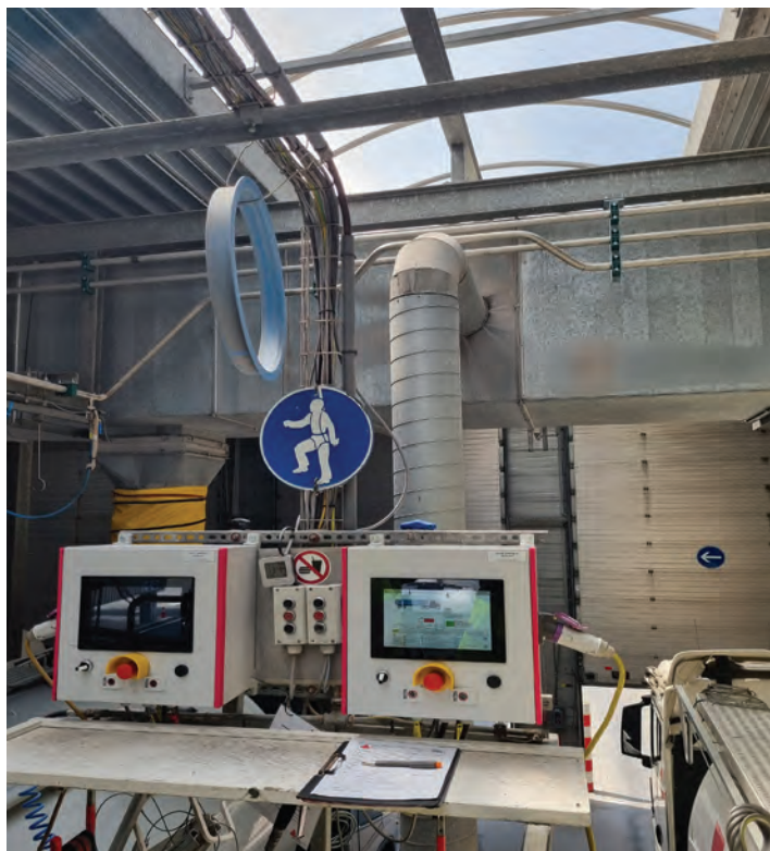
Upgraded PLC control at Katoennatie
